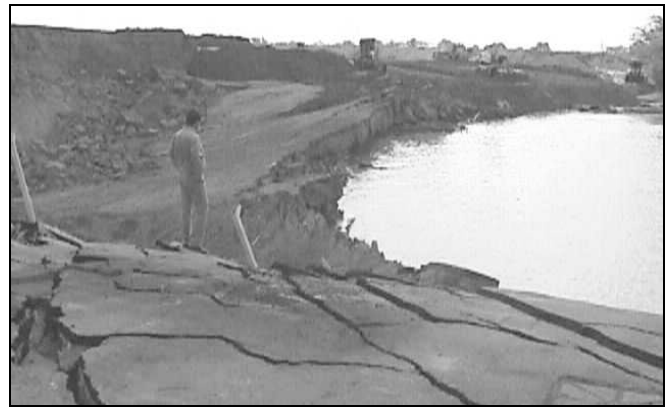
Figure 4. Sliding mass as seen from the wharf.
